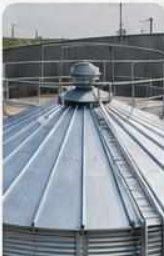
ROOF VENTILATION SYSTEM
